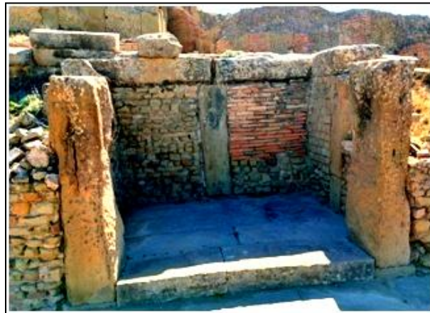
Figure 5: Example of brick usage in the repair of a wall in Timgad (source: Author 2023).
