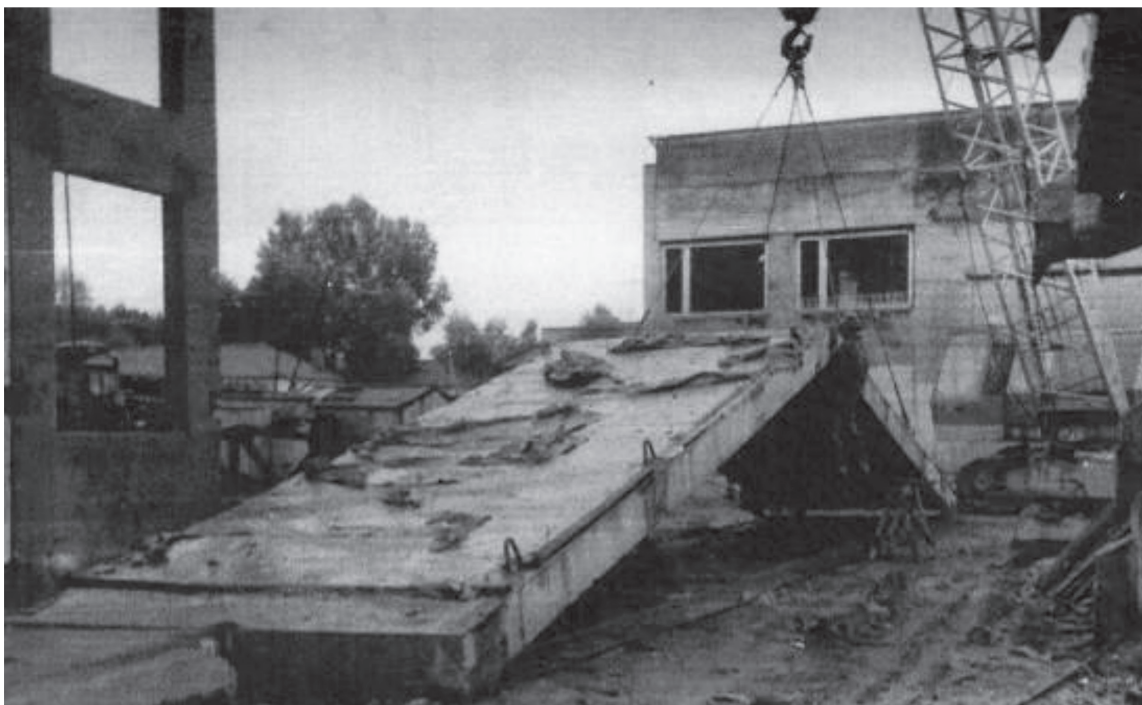
Fig. 5 Enlarging assembly of the covering panel and tensioning of the brace on the construction site
