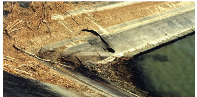
Fig. 8 Failure of the bituminous concrete facing of the Morávka Dam in 1996 (VD-TBD, 2021)
