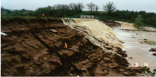
Fig. 6 Overtopping of the Pocheň Dam during the flood in 1996 (VD-TBD, 2021)
