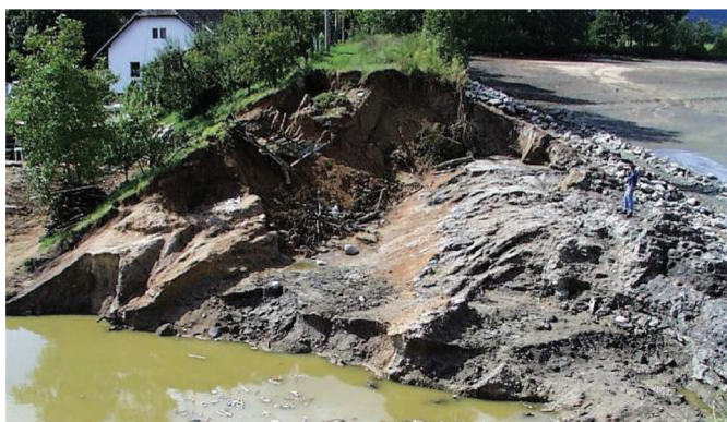
Fig. 3 The breached Metelský Dam (photo by authors)
