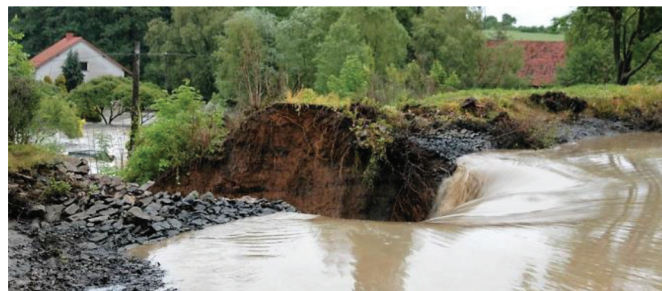
Fig. 5 The breach in the Mlékovice Dam during the 2013 flood (Švarc, 2014)
