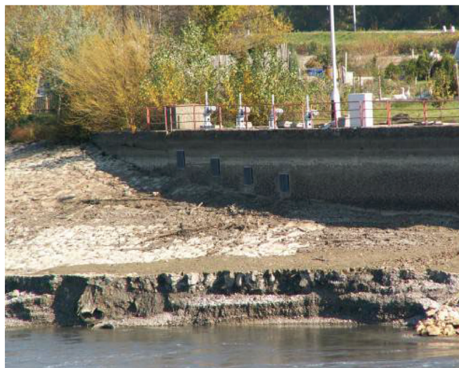
Fig. 1 The Váh cascade – the Drahovce water structure, inflow windows at different levels with control gates (photo from 2007, when the reservoir was empty)
