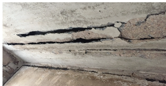
Fig. 1 Two sections showing the complete destruction of the protective layer of concrete with a length of l = 2400 \times 1360 mm and a width of a = 77 \times 72 mm, respectively
