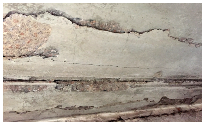
Fig. 3 An area showing the falling off of the surface layer of the concrete (part of the concrete layer is hanging down), S_{\text{area}} = 0.32 m 2 (pink color of concrete). The crack in the protective layer of the concrete has a length of l = 1440 mm and a width of a = 2.6 mm
