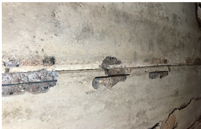
Fig. 4 Areas showing the destruction of the protective layer of the concrete, S_{area} = 0.04, 0.07 and 0.065 \text{ m}^2 , respectively, and the exposure of the working reinforcement (in the middle section, there are traces of soot on the reinforcement)
