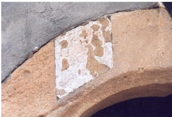
Fig. 2 The application of improper kind of sandstone
