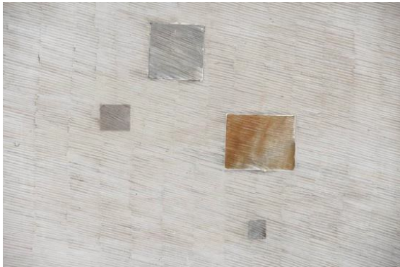
Fig. 1 The application of improper kind of sandstone
