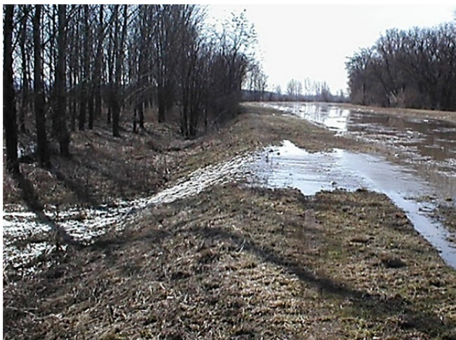
Fig. 1. Levee overtopping, to some extent similar to the flow over a broad-crested weir.
