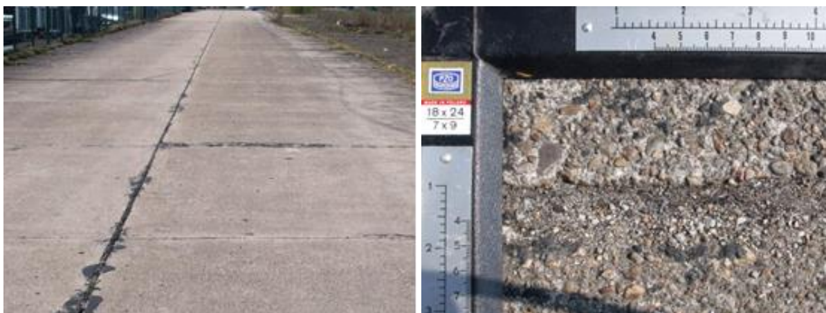
Figure 2 The road of the concrete slabs on the terrain of the old airport
