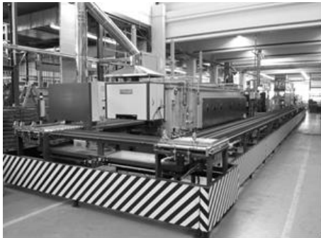
Fig. 5 Continuous belt sintering furnace (courtesy Mahler GmbH)
