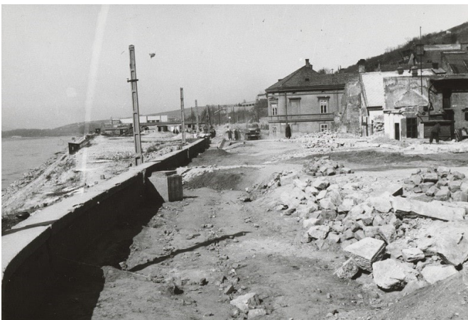
Fig. 4. Construction of the embankment. Photo: Pavol Poljak. (Source: Slovak National Gallery, after 1945)
