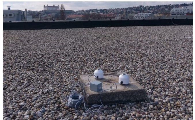
Fig. 6. Set of two pyranometers and a data logger on a roof. (Photo: Authors)
