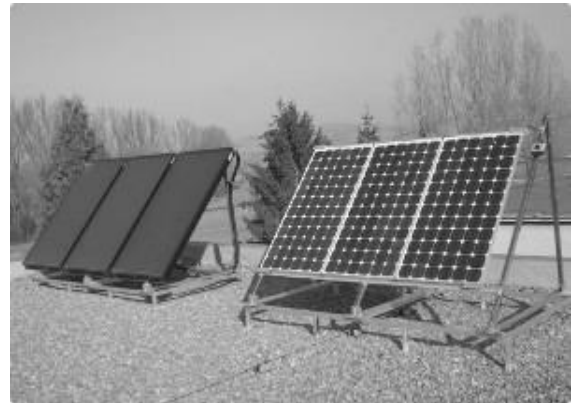
Figure 3 Solar and photovoltaic panels located on the roof of the centre building
