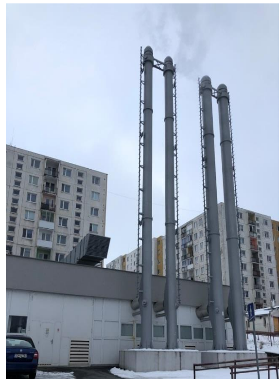
Figure 5 View of boiler room with CHP
