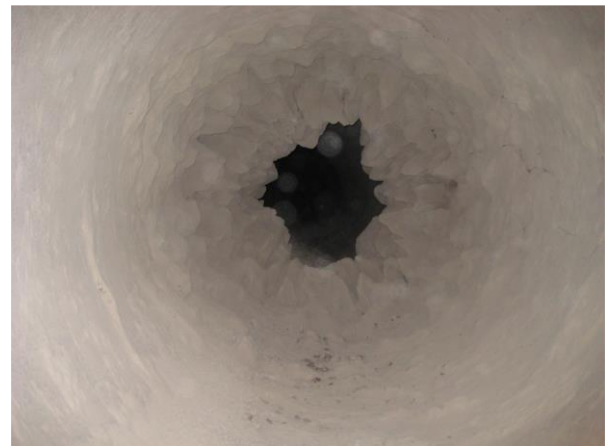
Figure 1 Ash ring in lime rotary kiln
