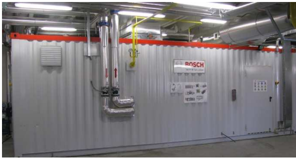
Figure 5 Container with cogeneration unit
