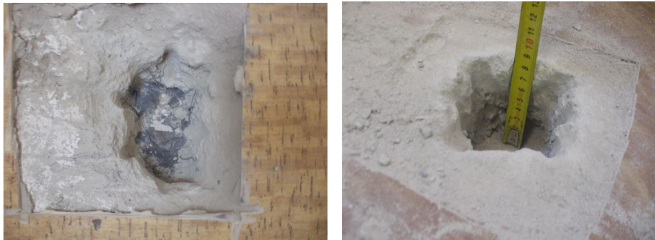
Figure 8: Probe to determine the thickness and composition of the floor on the ceiling panels
