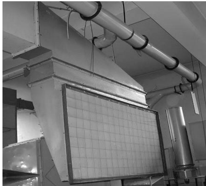
Figure 1: Stand for studying the air velocity field of the double-equal strength inlet device (double-exponential profile) for spatial air-distribution.
