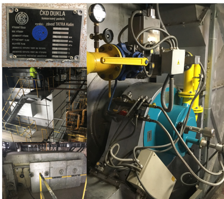
Figure 3. Boiler OK 60 ČKD Dukla. Clockwise: one of 4 gas burners; the top of the boiler duct; height view of the boiler; label with technical parameters of the boiler.
