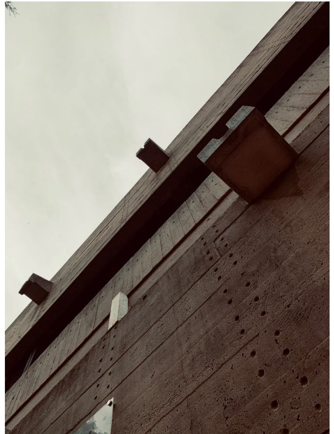
Fig. 12.4. Concrete details and finishes, meticulously crafted to assist in proper drainage. (Photo: Cornelius van der Westhuizen, 2022)
