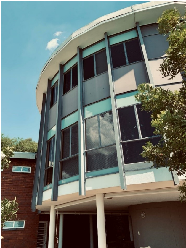
Fig. 9.1. The Round House exterior detail, the asbestos and steel facade is put on display. (Photo: Cornelius van der Westhuizen, 2022)
