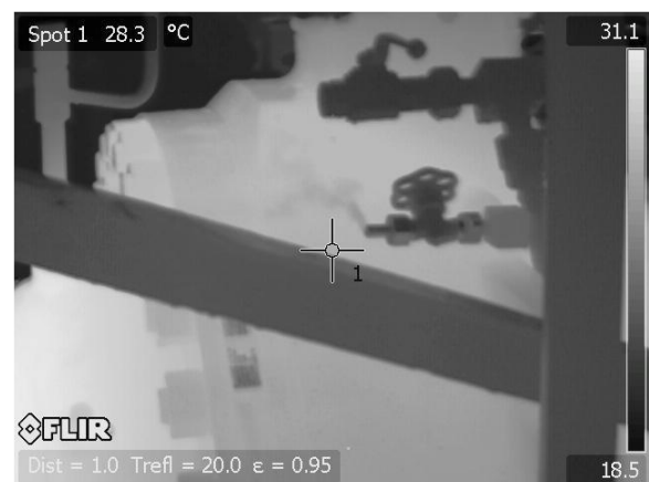
Figure 1 Identification of natural gas leaks.
