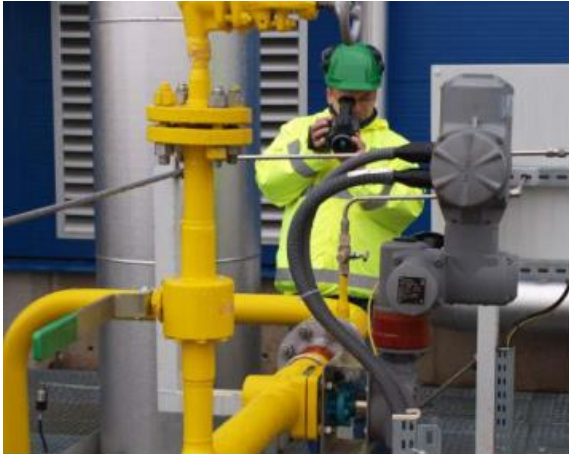
Figure 2 Localization of gas leaks
